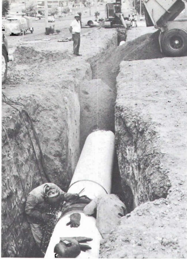
Laying the Gas and Fuel Corporation's 30 inch Dandenong to West Melbourne natural gas pipeline along Dandenong Road, Clayton in October 1969.
